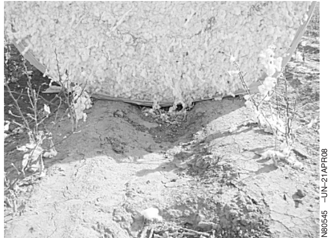
Incorrect Staging Surface Figure A
